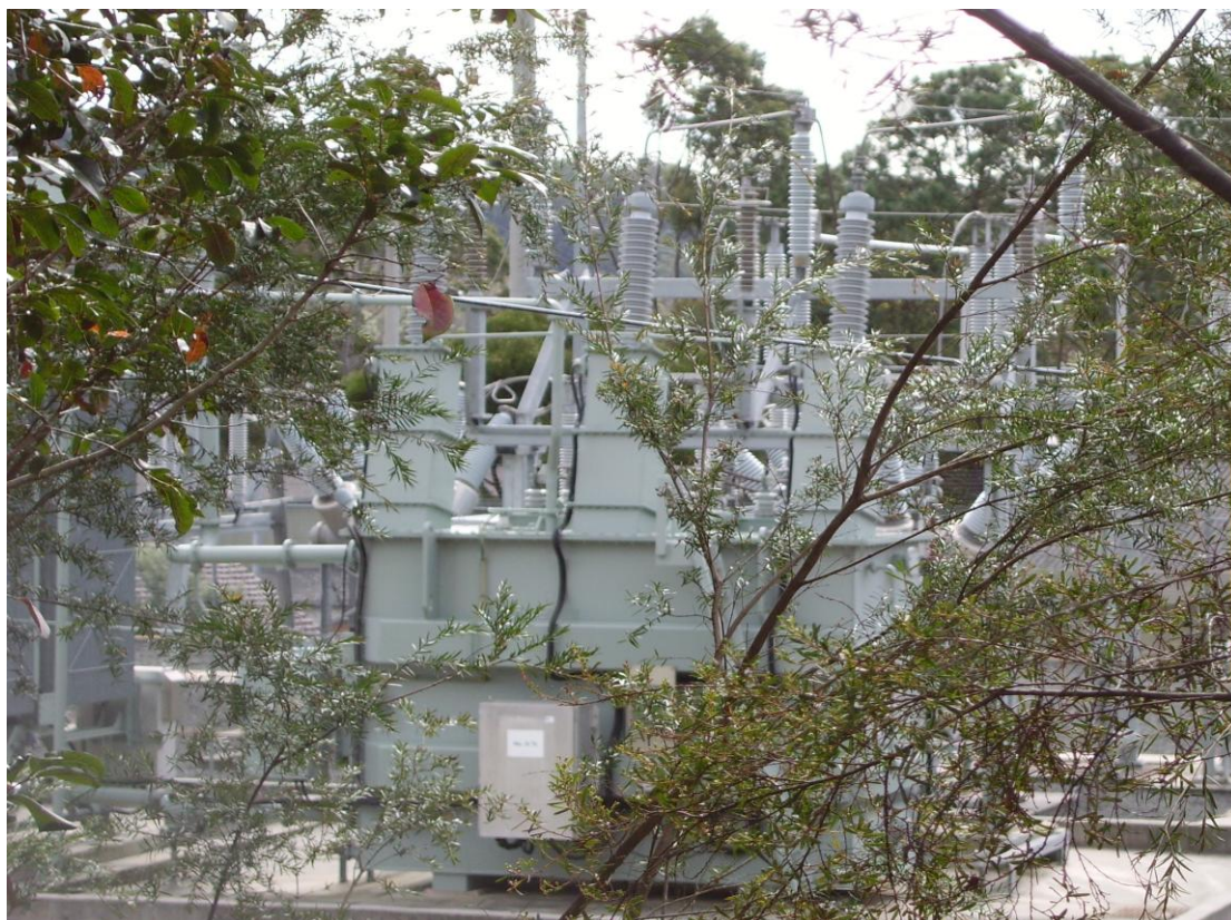
Photo: Electrical Sub-Station at West Gosford
